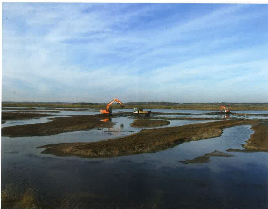
← Re-profiling nesting islets on Havergate Island, allowing occasional flooding to control vegetation and rats, and to create better visibility for visitors. Smaller equipment was used here because of the size and weight constraints of the vehicle ferry used for transport. Kieren Alexander/RSPB
